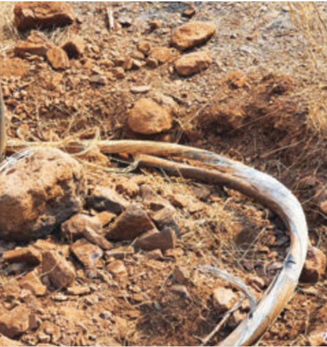
These damaged cables caused the power outages.
